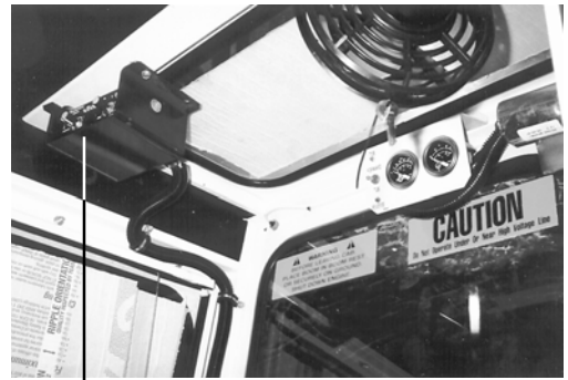
location of the electronic governor on an HD-12 equipped with a grapple loader
